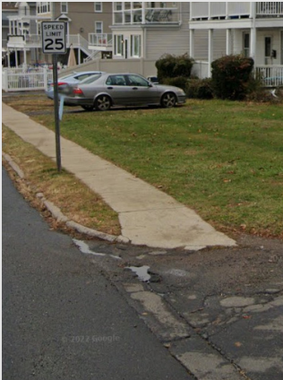
Non-Compliant ADA Ramps
