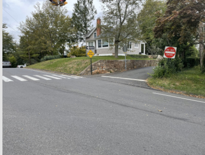
Non-Compliant Ramp Across Shore Drive to Clark Avenue
