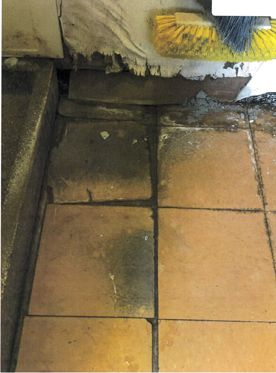
Leak from ground floor water closet (repair in progress); tile floor may need abatement
