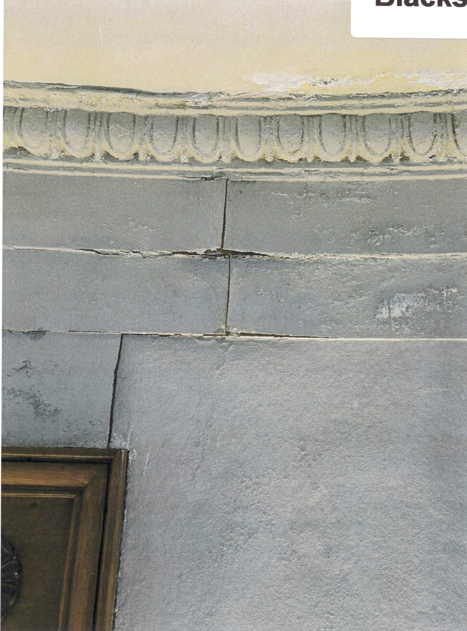
Plaster crumbling, First Floor mezzanine wall/ceiling around curved section
