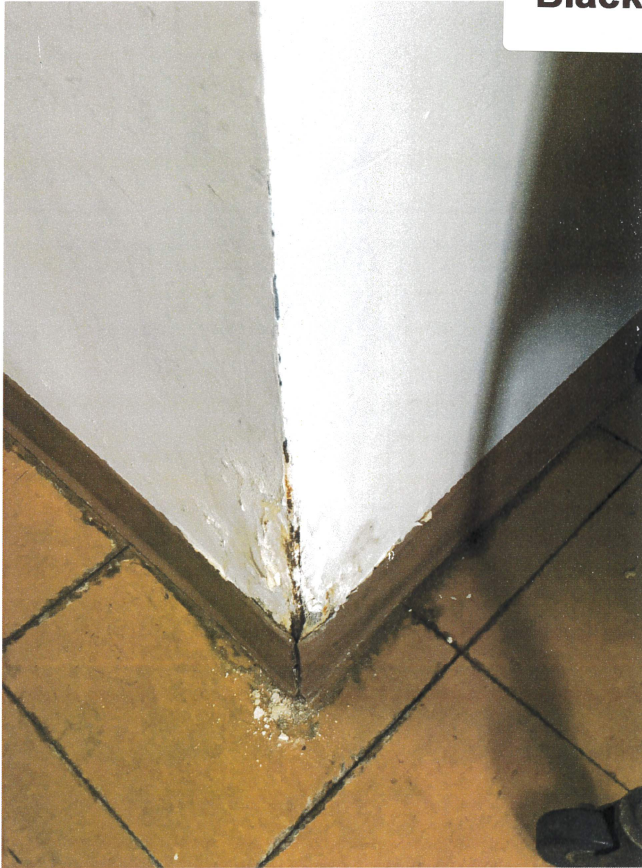
Leak from ground floor water closet (repair in progress); tile floor may need abatement
