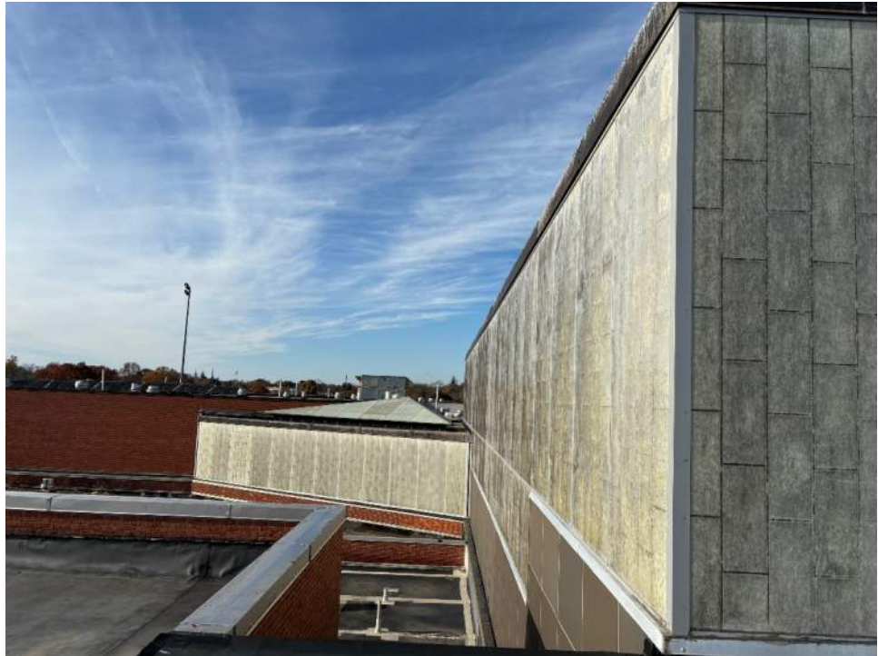
View looking east towards Roof 2 skylight and translucent wall panel. Roof 14 translucent wall panel is visible on the right.
