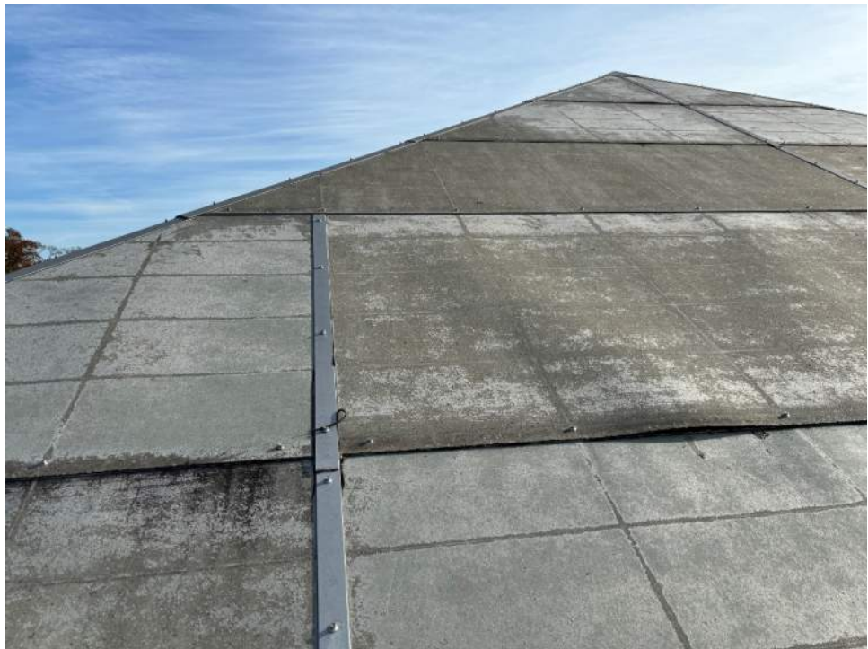
Close up of large skylight. Note the fading, delaminating, and gaps.
