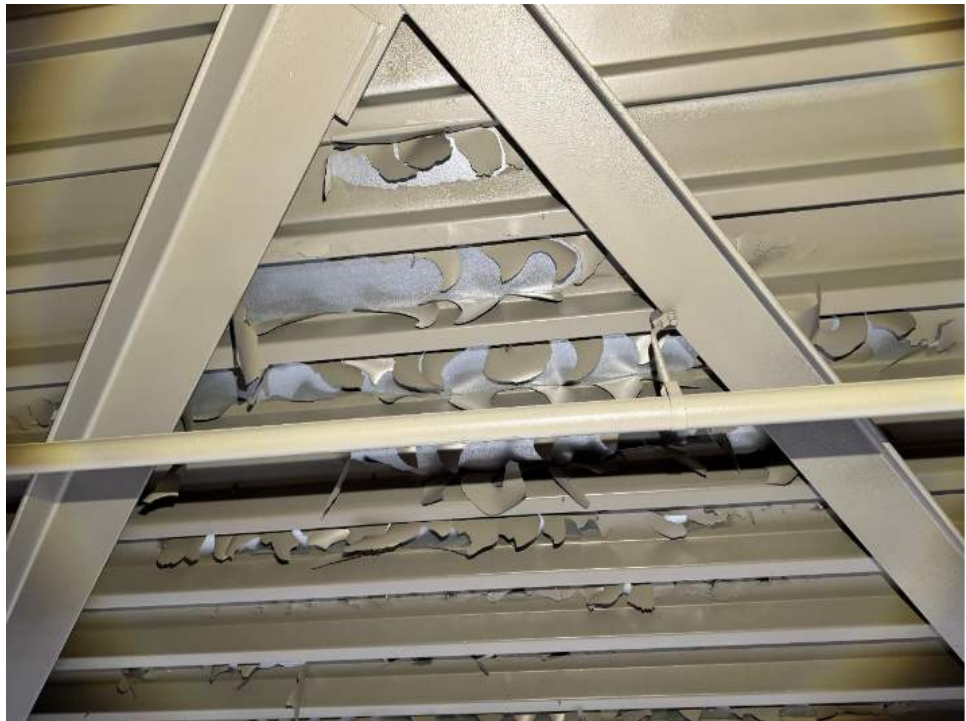
Interior view closeup of peeling paint at roof deck
