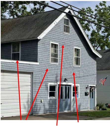
leaky windows & doors
