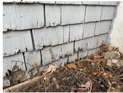
deteriorating shingles below grade
